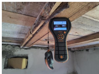
Overflate himling - Fuktmåling i himling.
