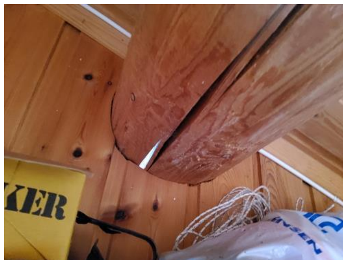
Overflater himling - [Sprekker i drager]
